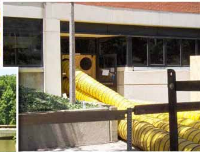
(ABOVE) Large yellow tubes pump hot air into the east side of the BCSB basement to accelerate the drying process. Five feet of water spilled into the building from the nearby Iowa River during the city's worst flood since 1851.
